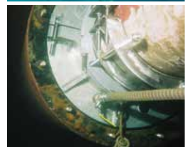
Above: The inflatable habitat is fitted around the stern seal area creating a water tight fit (top) and a blanking system for repair/replacement of internal face seals (below).
