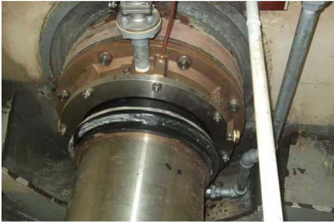
Figure 8. Installation of forward axial seal
