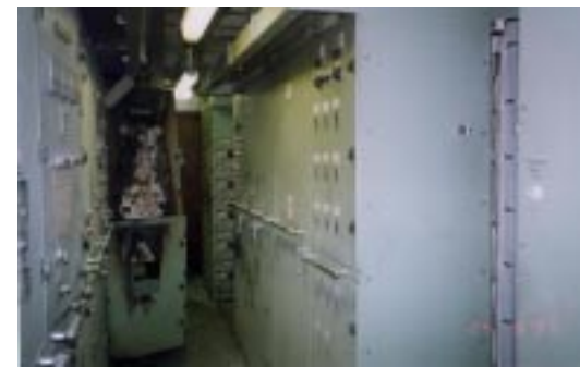
View of main switchboard room
