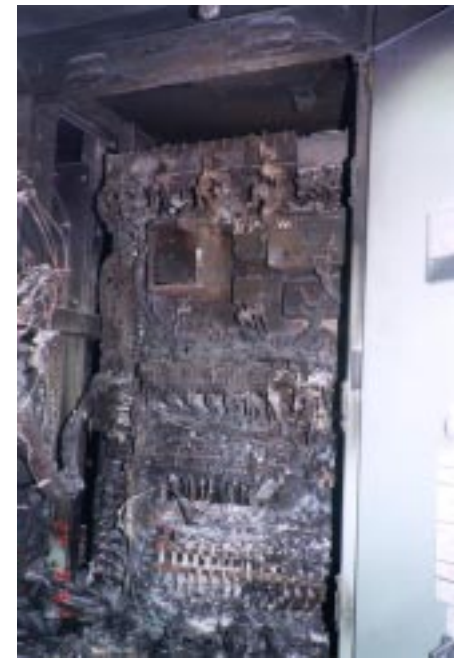
Fire damage No.2 D/G upper level
