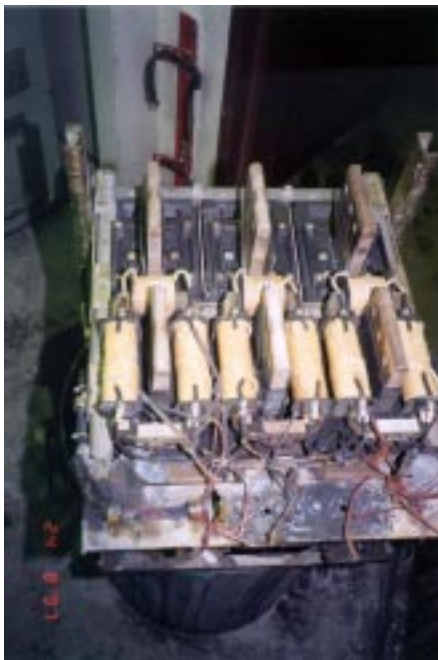
Fire damage No.2 ACB back C.T.'s on outgoing lines
