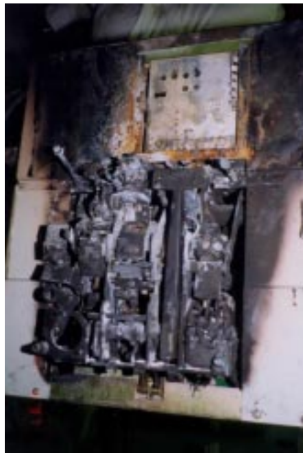
Fire Damage No.2 ACB view
