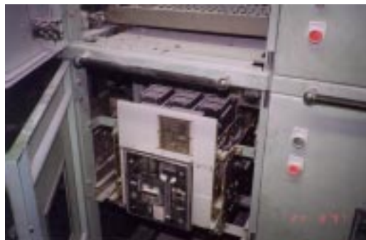
Hyundai type circuit breaker
