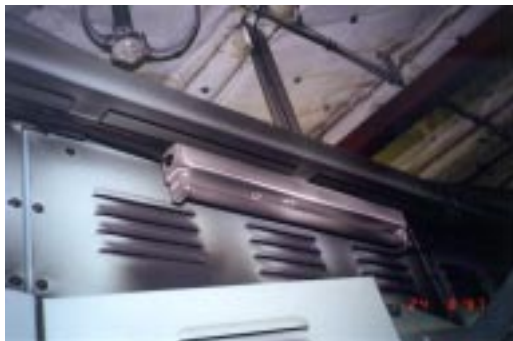
Heat detector above synchronising panel
